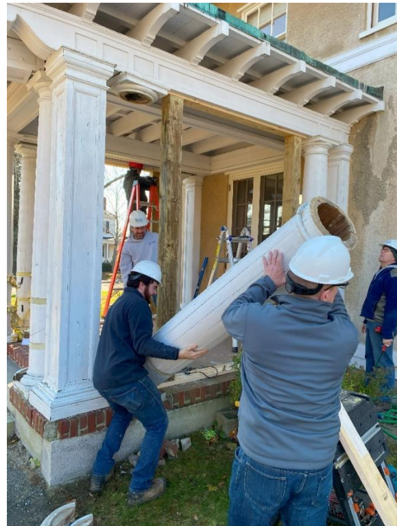
Restoration of the port cochere at the First Amendment Museum in Augusta required careful removal, repair, and reinstallation of original wood columns. Photo: First Amendment Museum
