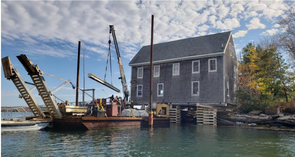
The Queen Mary, a building integral to the National Audubon Society's historic Hog Island Camp in Bremen, was structurally reinforced and raised three feet on new pilings in response to rising seas and more intense weather events due to climate change. Photo: National Audubon Society
